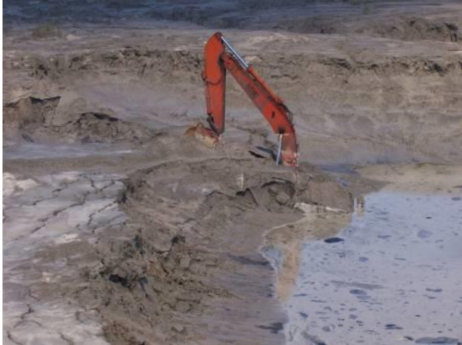
Figure 1.16: Side picture of Trackhoe covered with fly ash caused by fly ash failure at the DPL impoundment
