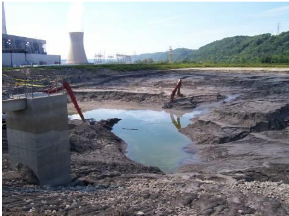
Figure 1.17: Portion of a fly ash flow failure in an impoundment at the DPL power plant
