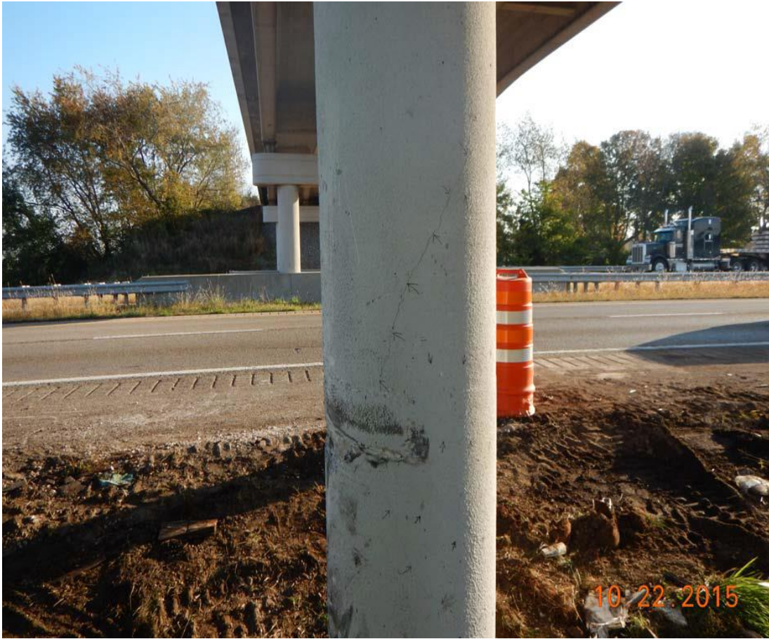
Figure 5.13- Spalling and cracks observed at the point of impact
