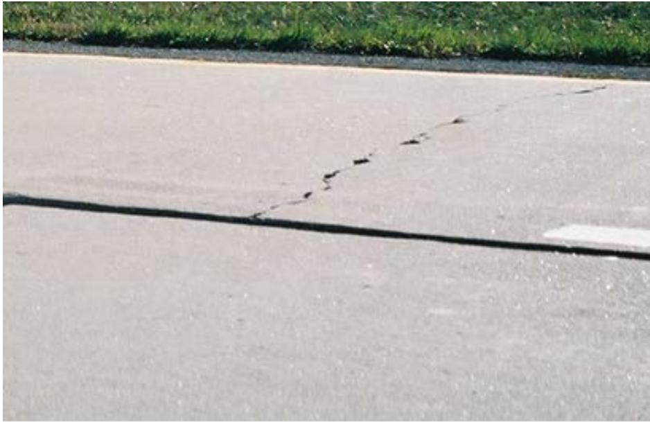
Figure 8. Typical PCC transverse cracking
