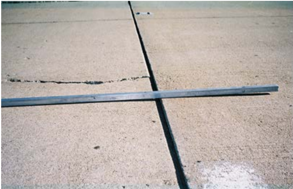
Figure 9. Typical PCC joint faulting
