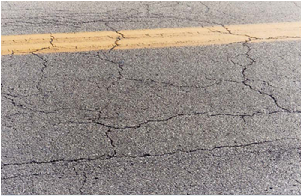
Figure 7. Typical HMA thermal (block) cracking
