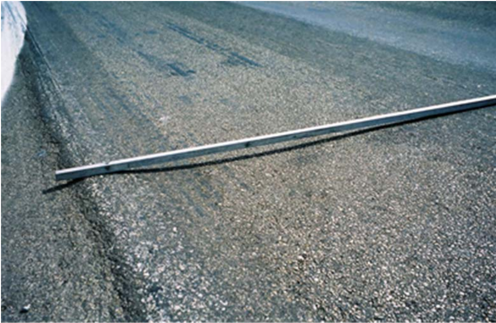
Figure 5. Typical HMA rutting
