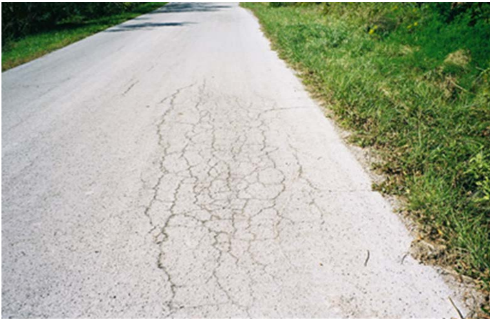
Figure 6. Typical HMA fatigue cracking
