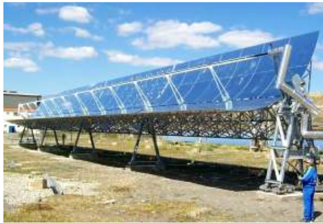
Fig. 2.5: Photograph of an installed EuroTrough parabolic trough system [26].
