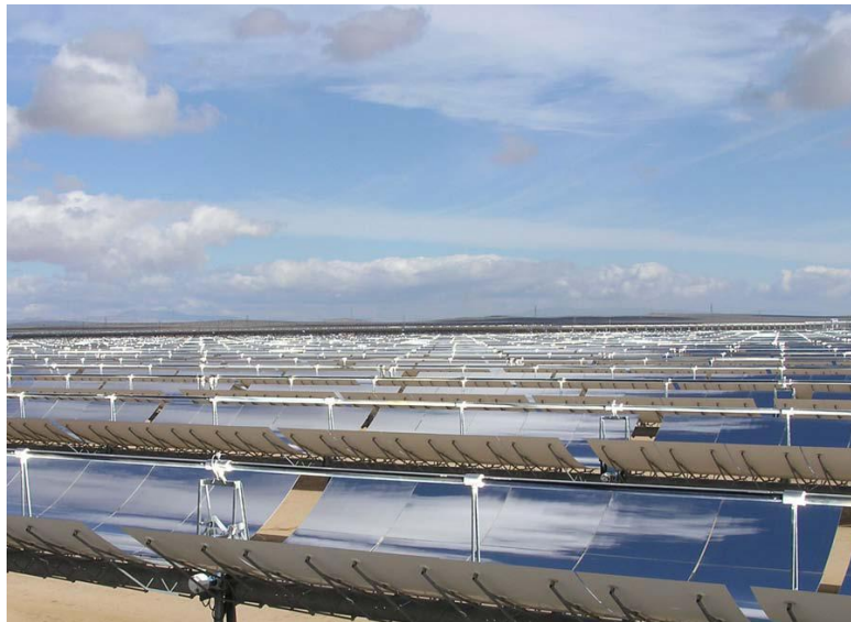
Figure 1.2: 30 MW parabolic trough Solar Energy Generating Systems (SEGS) plant in Kramer Junction, California [11]
