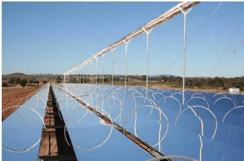
Figure 1.3: Compact linear Fresnel collector in Bakersfield, California by Ausra [11]
