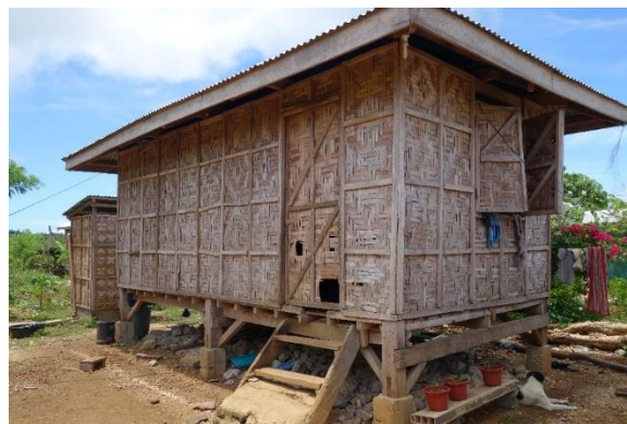
Shelter materials show signs of wear
