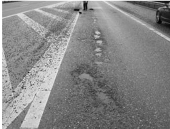
Figure 4.2: Frost damage on porous pavement (RWS 2012)
