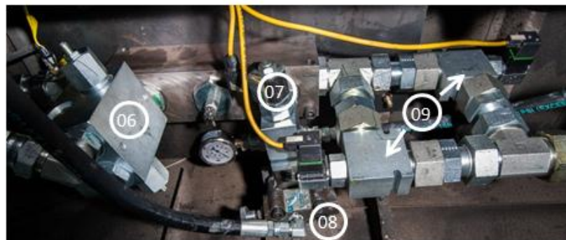
Figure C.3: Pictorial reference for the hydraulic components on the HHB
