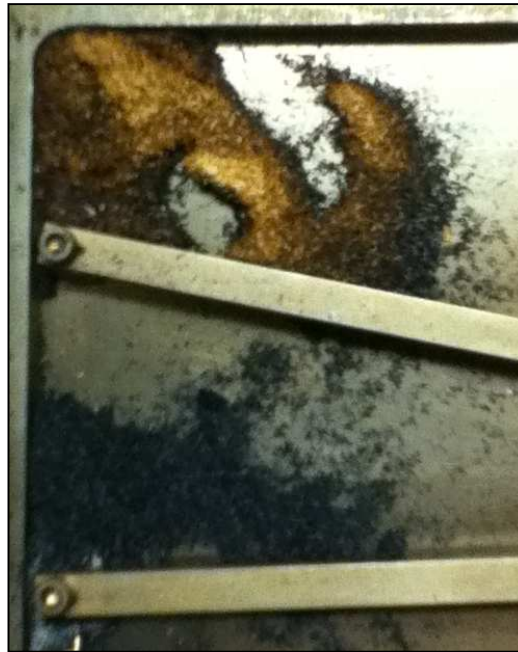
Figure 5.22- Buildup of Char and Torrefied Biomass on Upper Spreader During Early Commissioning Test
