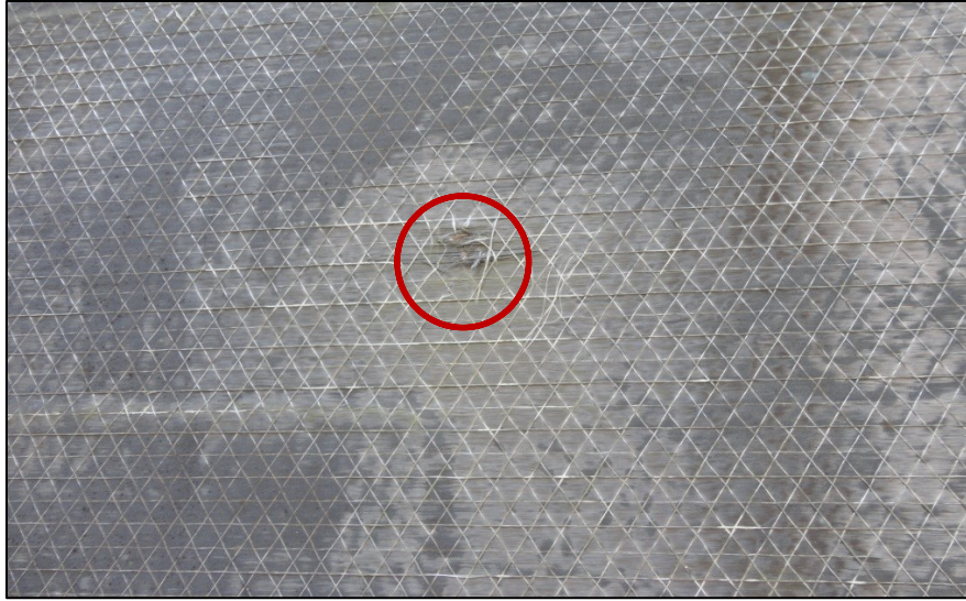
Figure 48: Tear in Fabric on North Side of Wall 3
