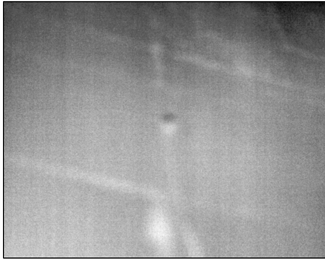
Figure A7: Thermal Image at Location 2 at 10:32 AM (North Side of Wall 2)
