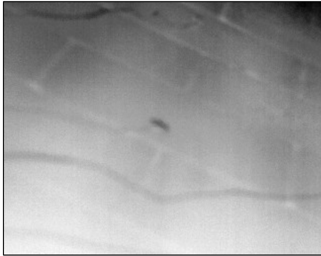
Figure A43: Thermal Image at Location 14 at 1:23 PM (North Side of Wall 2)
