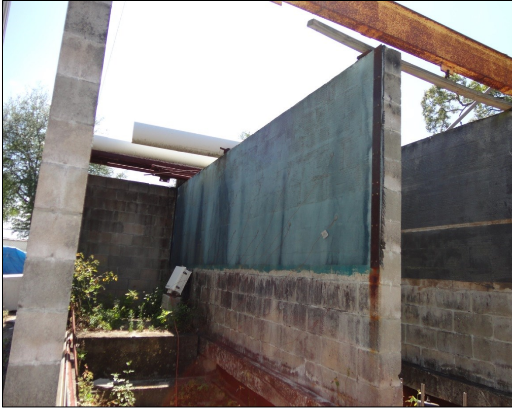
Figure 10: Thermocouples Installed on Wall 2
