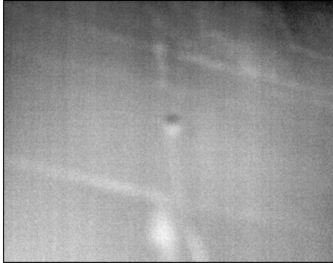
Figure 30: Thermal Image Location 2 10:32 AM (Wall 2 on the North Side)
