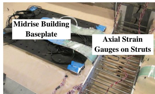
Figure 4-24. Excavation struts with axial strain gauges installed in the temporary excavation during model construction of E-Midrise.
