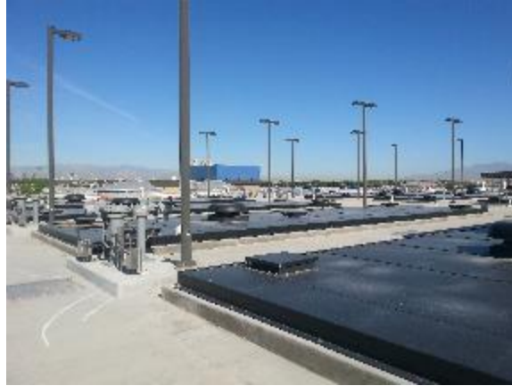
Figure 4.2: Full-scale filters at Clark County Water Reclamation Facility
