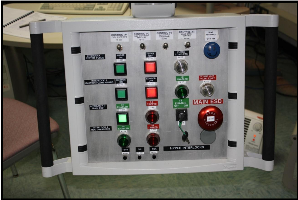
Figure 3.6: HyPer facility main control panel
