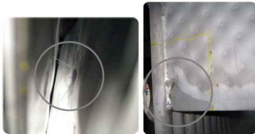
FIGURE 2.36 Leakage in a DSS 2205 evaporator due to vibrations or cyclic loads. [113]
