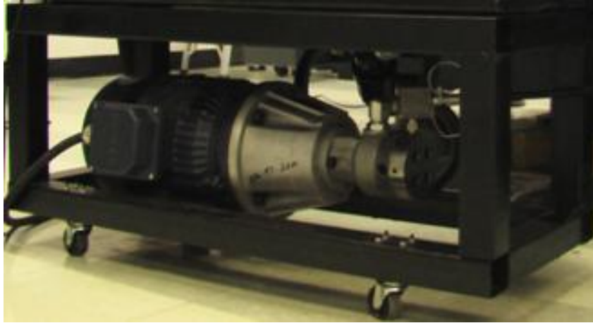
Figure 31: High pressure pump under reservoir tank
