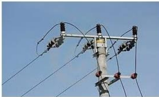
Fig. 2.2: Overhead power lines
