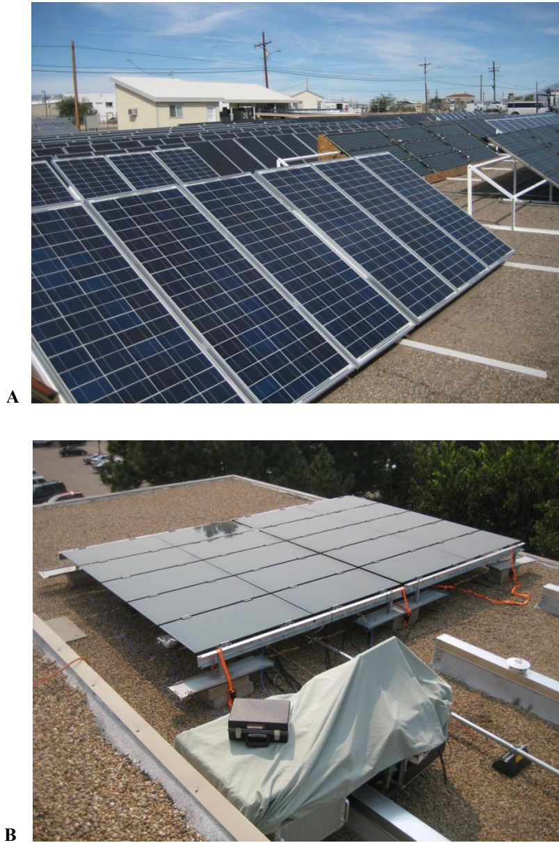
Figure 3.1. Ground mounted PV systems in Tucson, AZ (A) and roof mounted PV system in Boulder, CO (B)
