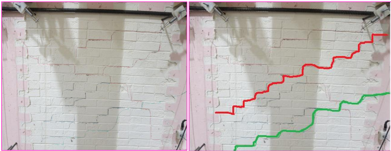
Figure 3-43. Nguyen CM Wall 1 shear cracks
