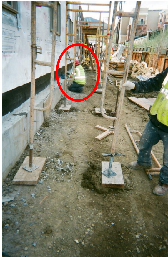
Figure 4.5: Bad Attitude Towards Criticism During Scaffold Installation Worker at ground level (inside red circle) ignored co-worker's request to move because scaffold was being installed and boards could fall off causing injuries.
