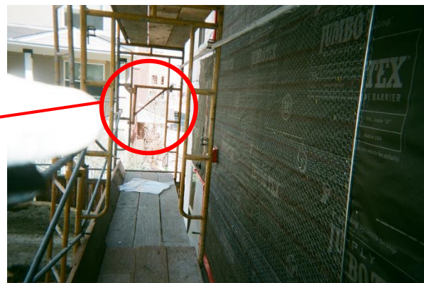
Figure 4.4: Scaffold Railing Improper
