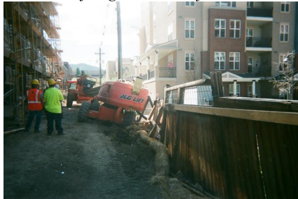
Figure 4.13: Forklift Near Scaffold
