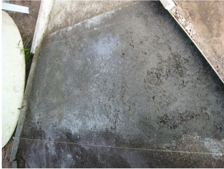
Figure 5.14 A thin strip of the entrance covered with sprinkles of Portland concrete cement.
