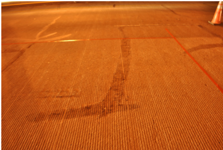
Figure 4-5 Residual "Crack-Chaser" Left on Deck
