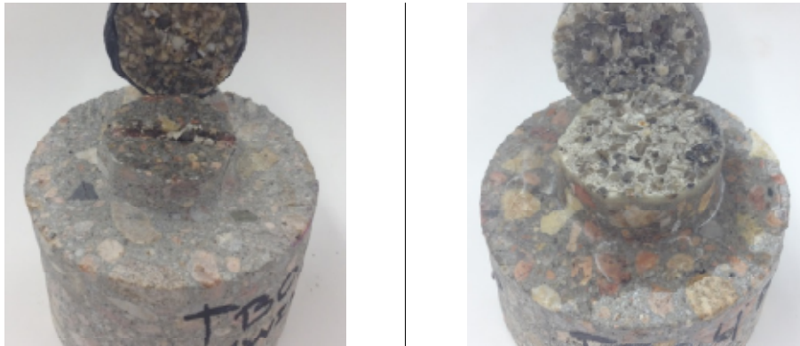
Figure 5-5 Polyester Class E & MMA Class O Failure Modes after 8 months of service
