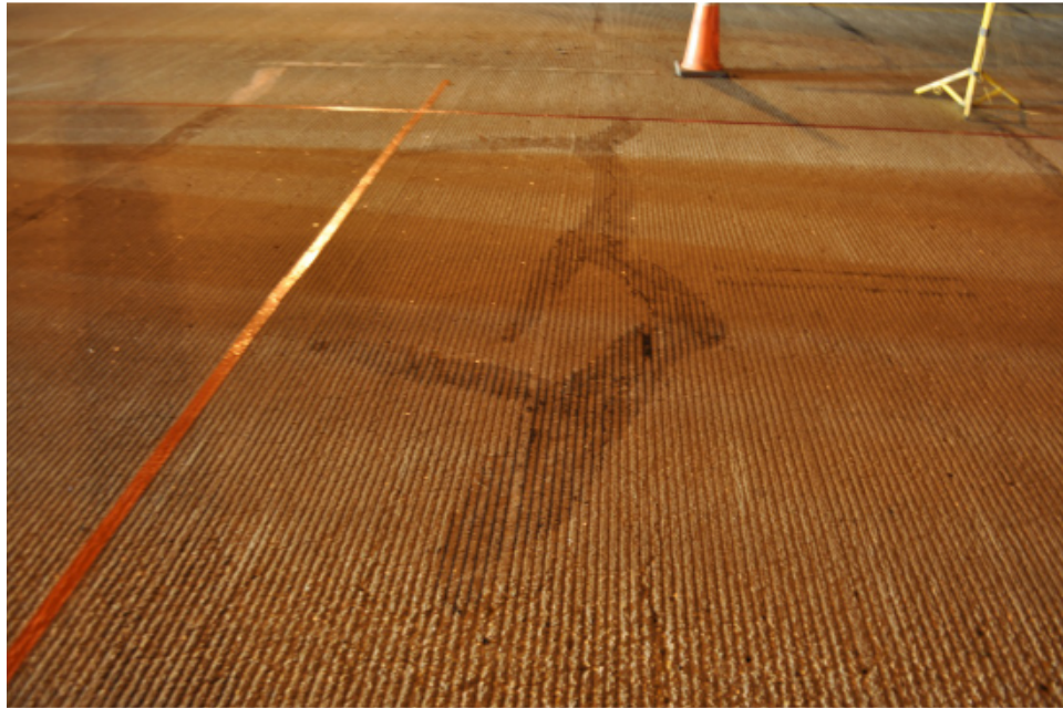
Figure 5-27 Residual crack chaser left on the deck
