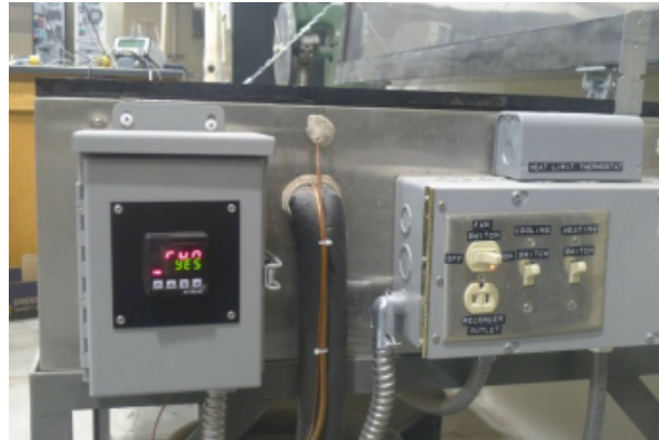
Figure 3-11 Digital Control Panels
