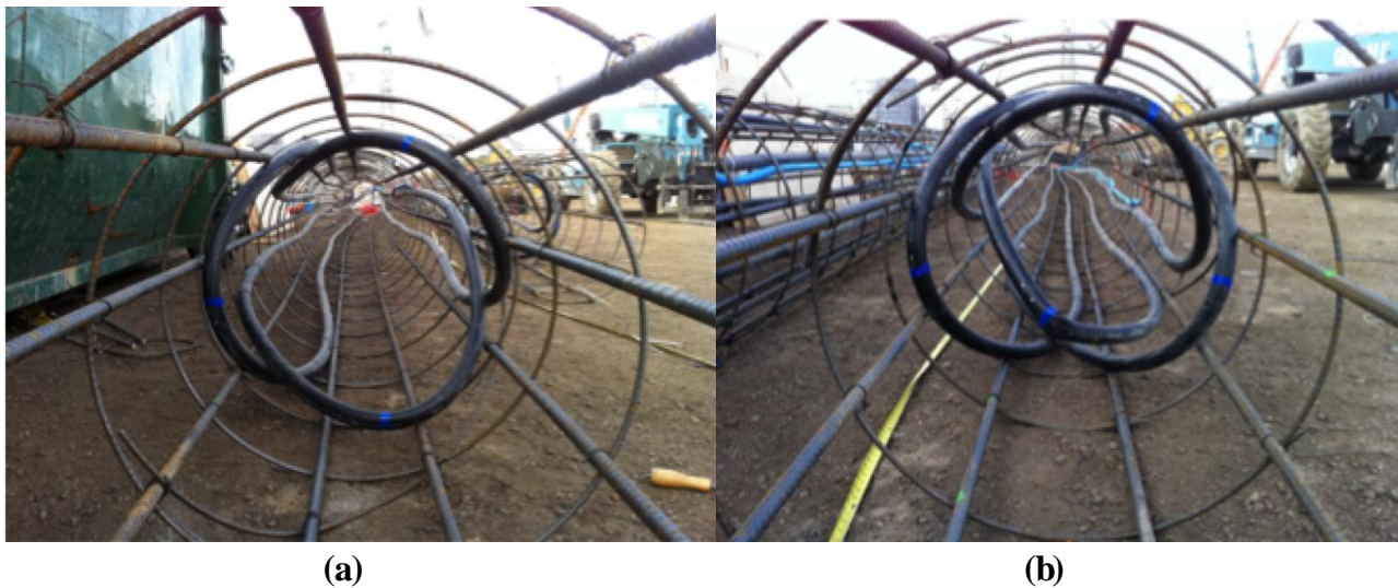
Figure 3.3: Heat exchanger tubing attached to reinforcement cages: (a) Foundation A, (b) Foundation B
