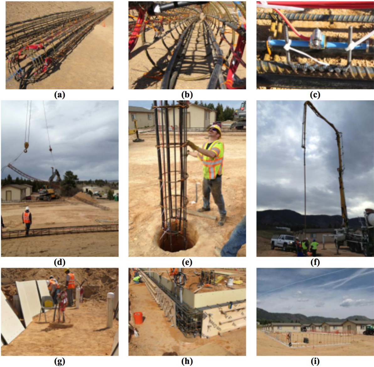
Figure 3.4: Construction photos: (a) Reinforcing cages with heat exchangers; (b) Inside view of cage; (c) Vibrating wire strain gauge; (d) Lifting with 3-point pick; (e) Lowering into uncased hole; (f) Concrete tremie; (g) Finished foundation; (h) Tubing in grade beam; (i) Completed grade beam and heat exchanger manifold
