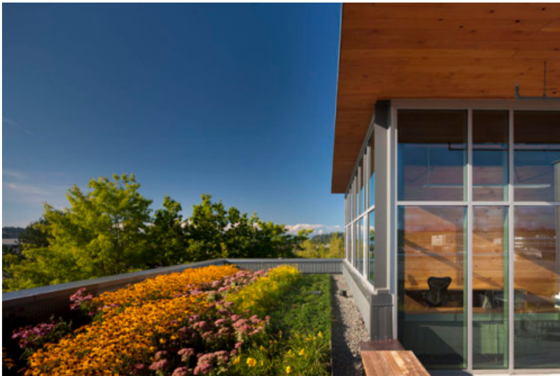
Figure 6.9: Vegetated Roof Accessible for Occupants – LOTT Clean Water Alliance
