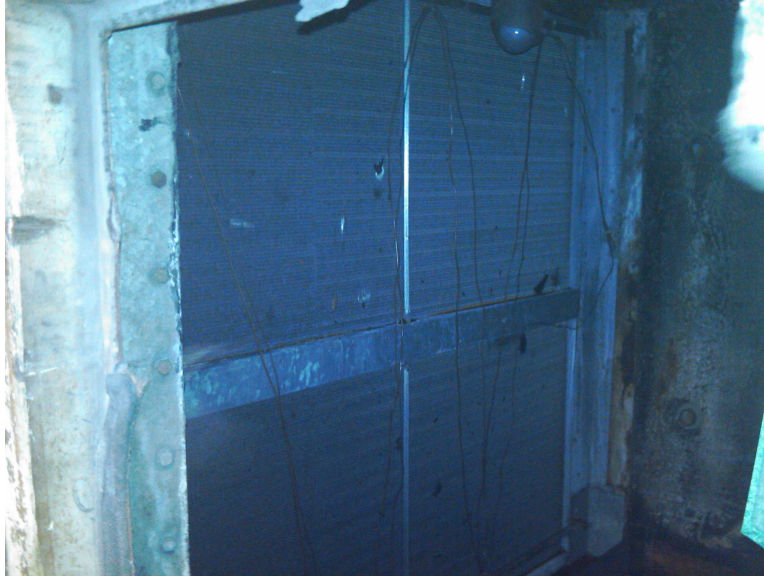
Figure 1 - MIT's AHU-6 coil detail
