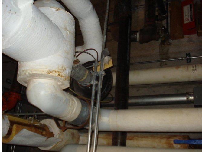
Figure 16 - Valve location near CUs AHU-6
