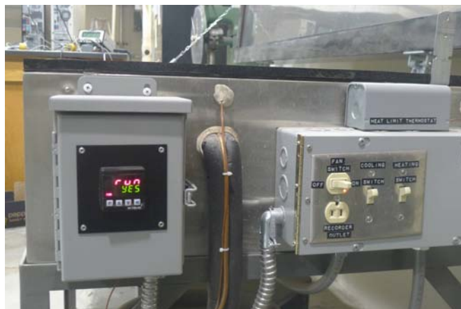
Figure 3.12 Digital controlling panels
