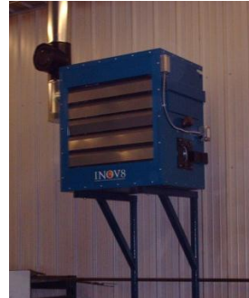
A.8: Industrial Shop Heater
