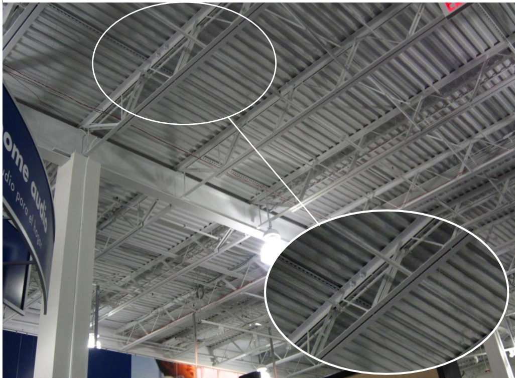
Figure 4.18 – Open web steel joist consisting of double angled chord members with alternating rod and double angled web members (Building 2).
