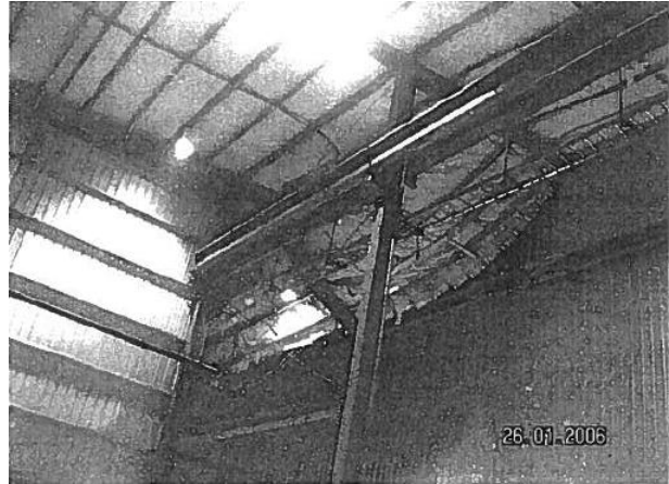
Figure 4.9 – Roof failure (J.R. Harris & Co. 2011).
