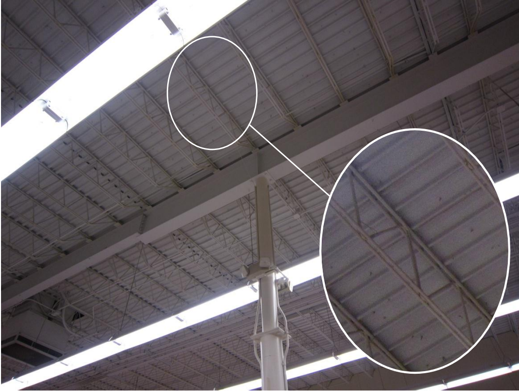
Figure 4.15 – Open web steel joist consisting of rods for web and chord members (Building 4).
