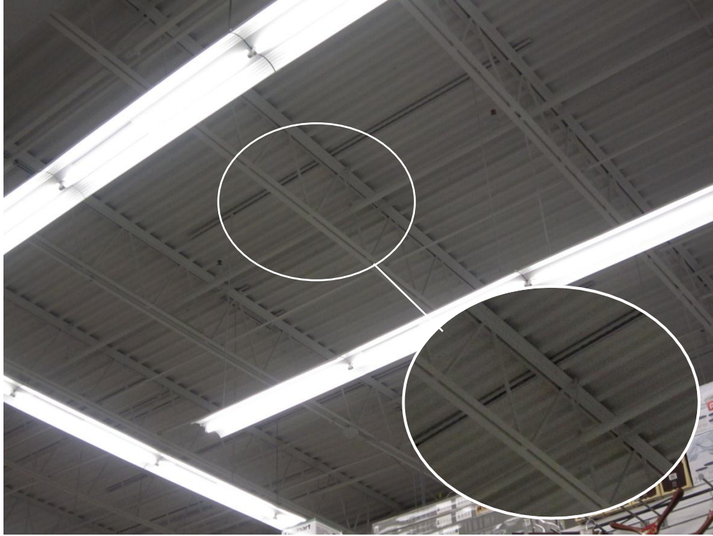
Figure 4.17 – Open web steel joist consisting of double angled chord members with rod web members (Building 1).
