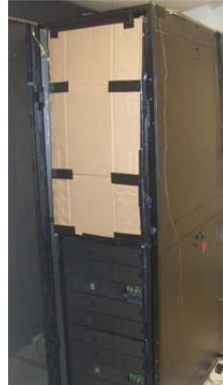
Figure 3–39: Top Servers Off and Blocked
