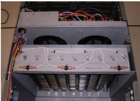
Figure 3–20: Server Simulator Heating Elements 21
