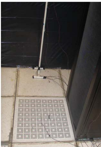
Figure 3–41: Rack Against the Perforated Floor Tile
