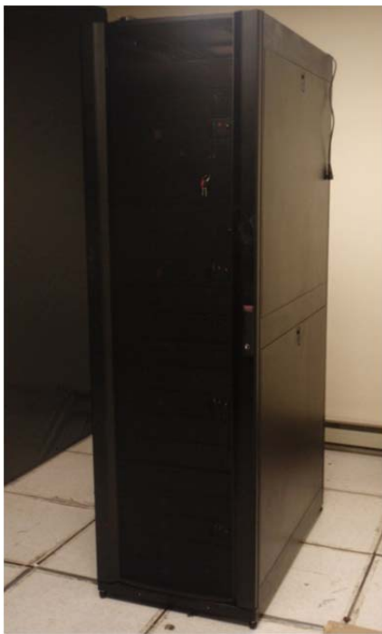
Figure 3–17: Rack with Server Simulators (Front View)
