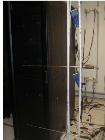
Figure 3–32: Anemometer Pole Set-up
