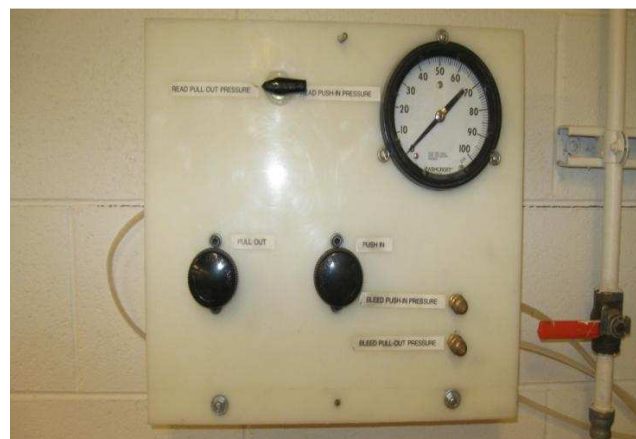
Figure 5.4 Control panel for the loading system (air pressure regulator).
