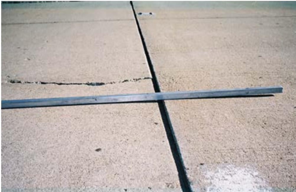
Figure 9. Typical PCC joint faulting
