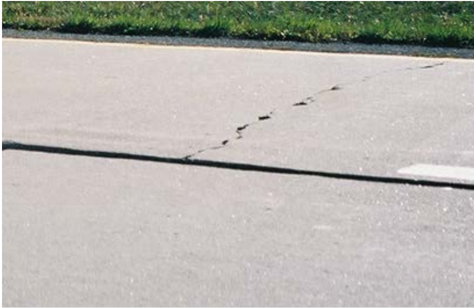
Figure 8. Typical PCC transverse cracking
