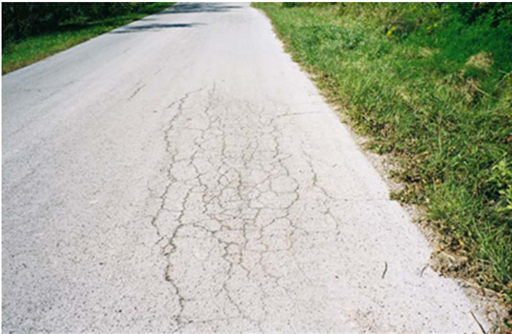
Figure 6. Typical HMA fatigue cracking
