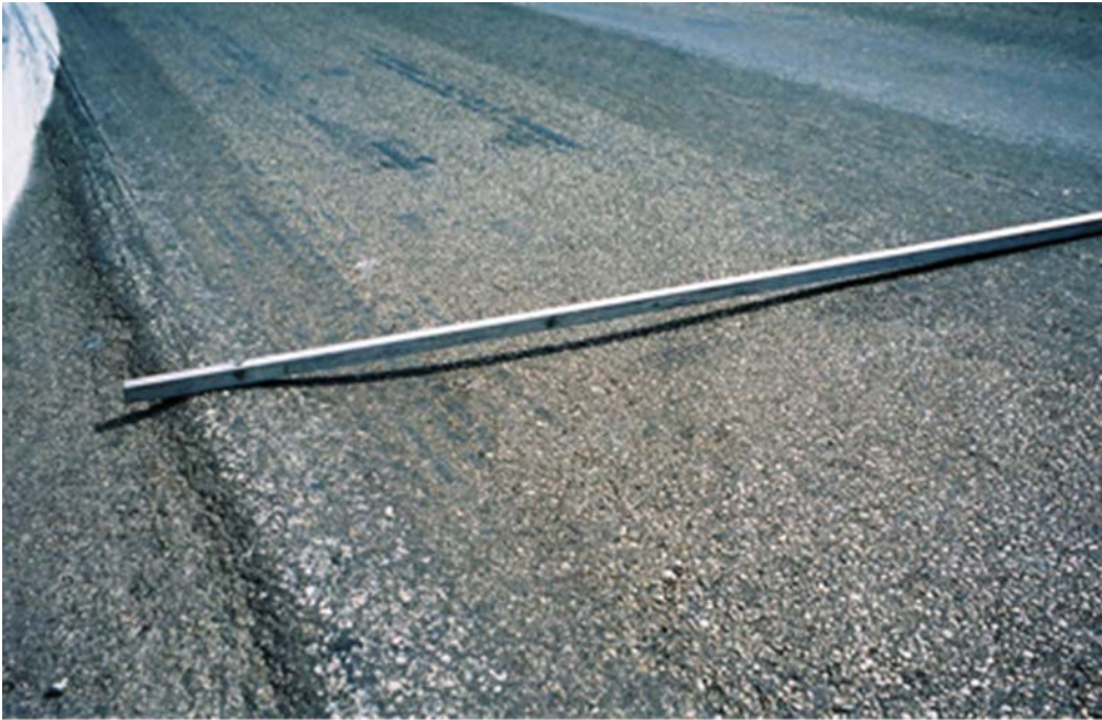
Figure 5. Typical HMA rutting
