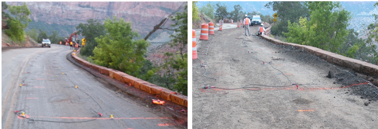
Figure 4.4. Layout of the 10 ft (3.0 m) geophone spacing at Zion N.P. grid #2 during (L) pre-grouting and (R) post-grouting seismic data collection.
