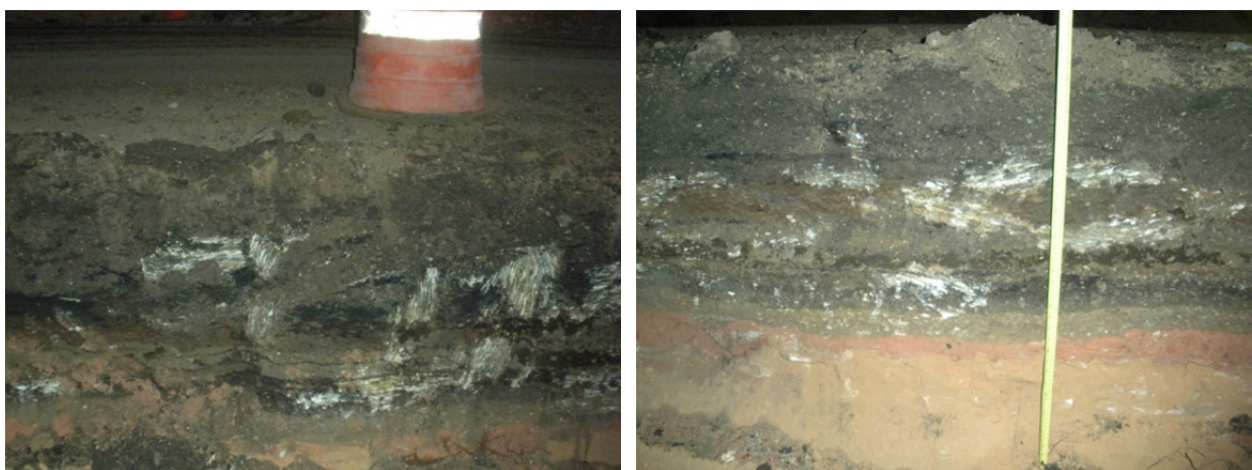
Figure 4.7. Asphalt thickness greater than 1 m (3 ft) observed at Zion N. P. site due to repeated maintenance patching to correct settlement.
