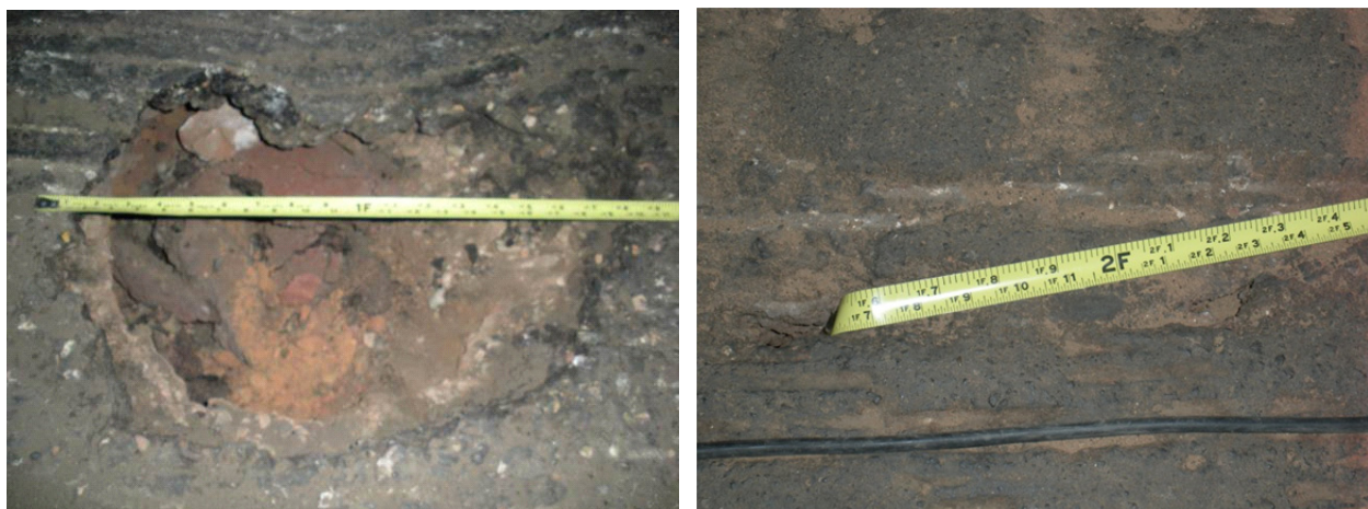
Figure 4.2. Voids beneath roadway surface daylighting at Zion N.P.: (L) Large void opening resembling a pothole, more than 0.5 m (1.5 ft) in width; and (R) small hole in pavement surface observed to open to a much larger void beneath pavement.
