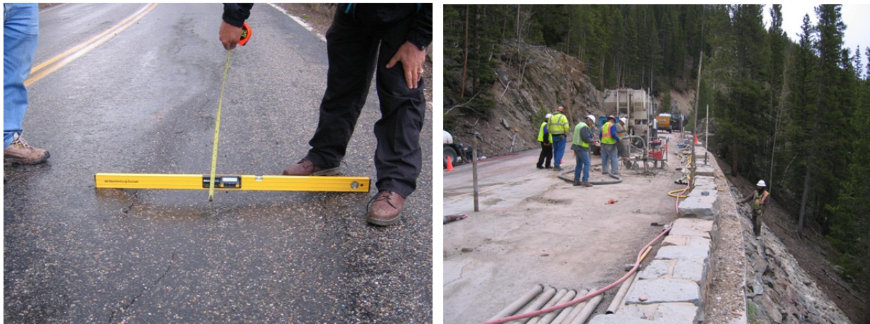
Figure 3.7. Photographs showing (L) differential settlement of roadway and (R) compaction grouting operations at Rocky Mountain N.P.
