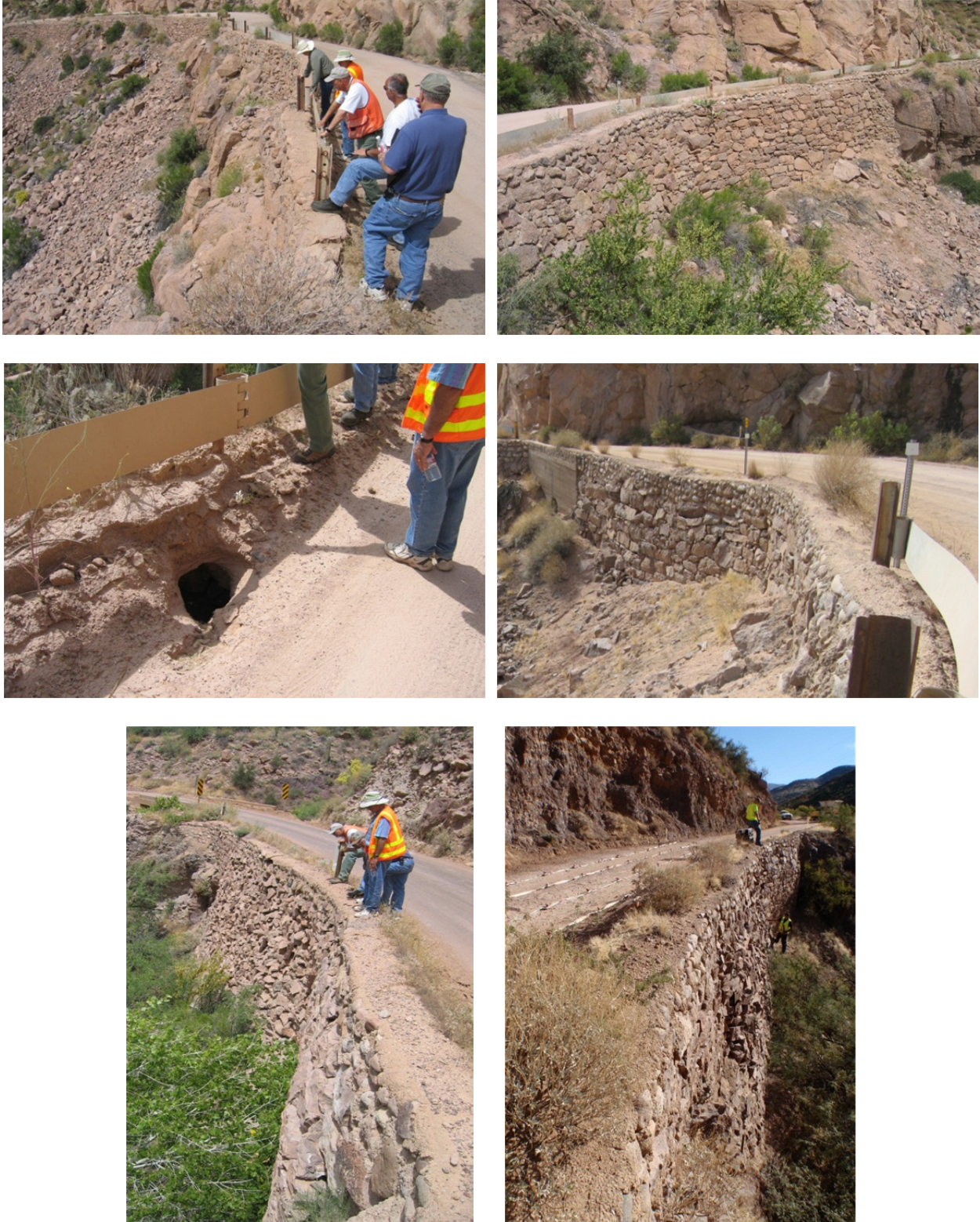
Figure 5.3. Photographs of Apache Trail retaining walls: clockwise from top left: (1) Location 1; (2) Location 2; (3) Location 3; (4) and (5) Location 5, Wall 1; (6) large void daylighting at the roadway surface at Location 4.
