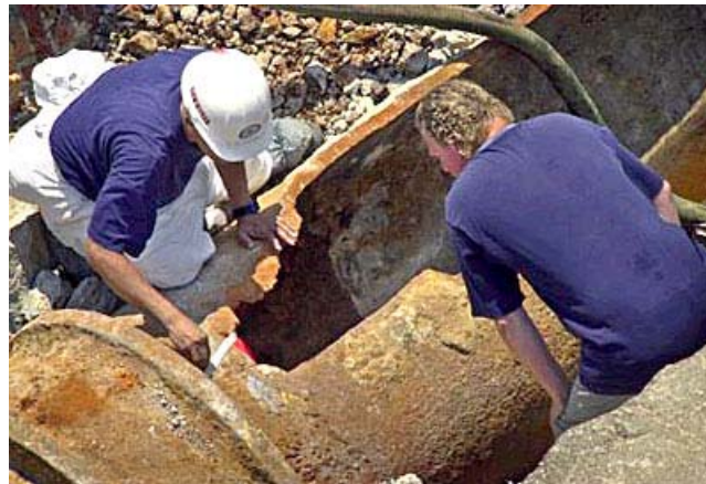
Figure 2.2: Ruptured 40-inch water main ( The Baltimore Sun 2001 )
