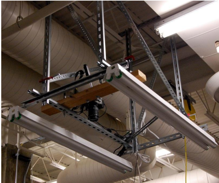
Figure 14: Top view camera, ceiling frame & auxiliary lighting.
