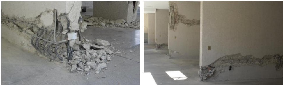
Figure 3-5. Damage due to concentration of vertical steel bars at end of walls (Leon, 2010)
