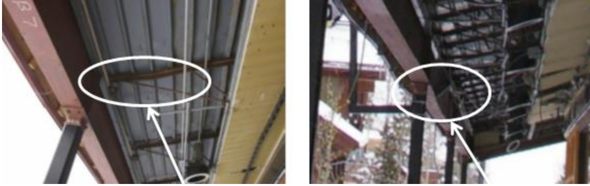
Figure 5.1- Deflected (a) bar joists and (b) wide flange beams due to large snow loads in February 2008 (Knott Laboratory 2008).
