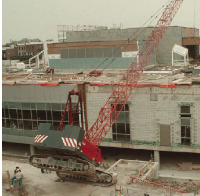
Figure 3: Tip-over Accident of a Mobile Boom Crane [10]
