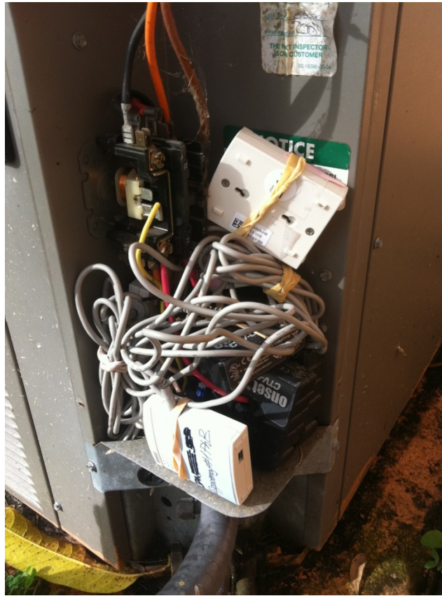
Figure 3-5 Data loggers and current transformers installed in the AC unit
