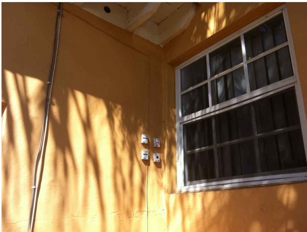
Figure 3-6 Outside temperature loggers installed on the west side of the house
