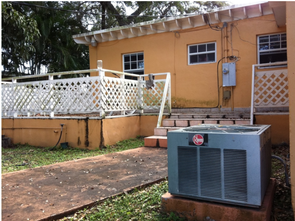
Figure 3-4 Rear of the experiment house and the air conditioner unit
