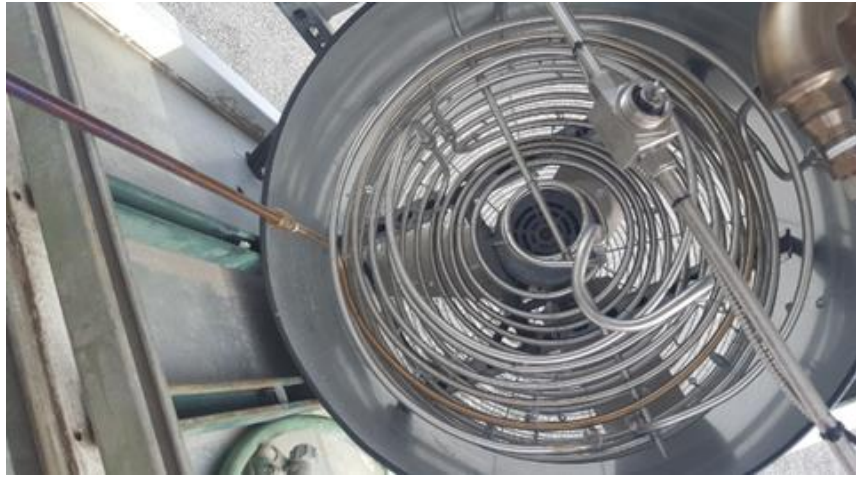
Figure 14. Air Cooled Heat Rejection Heat Exchanger
