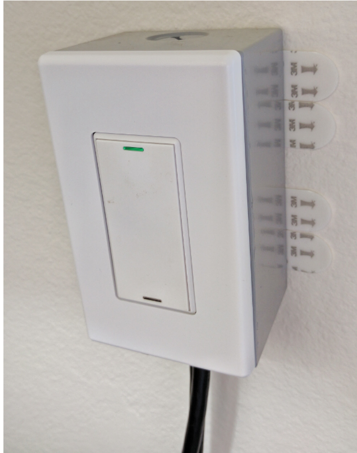
Figure 3.4: A ZigBee light switch is used to control devices and provide user feedback.
