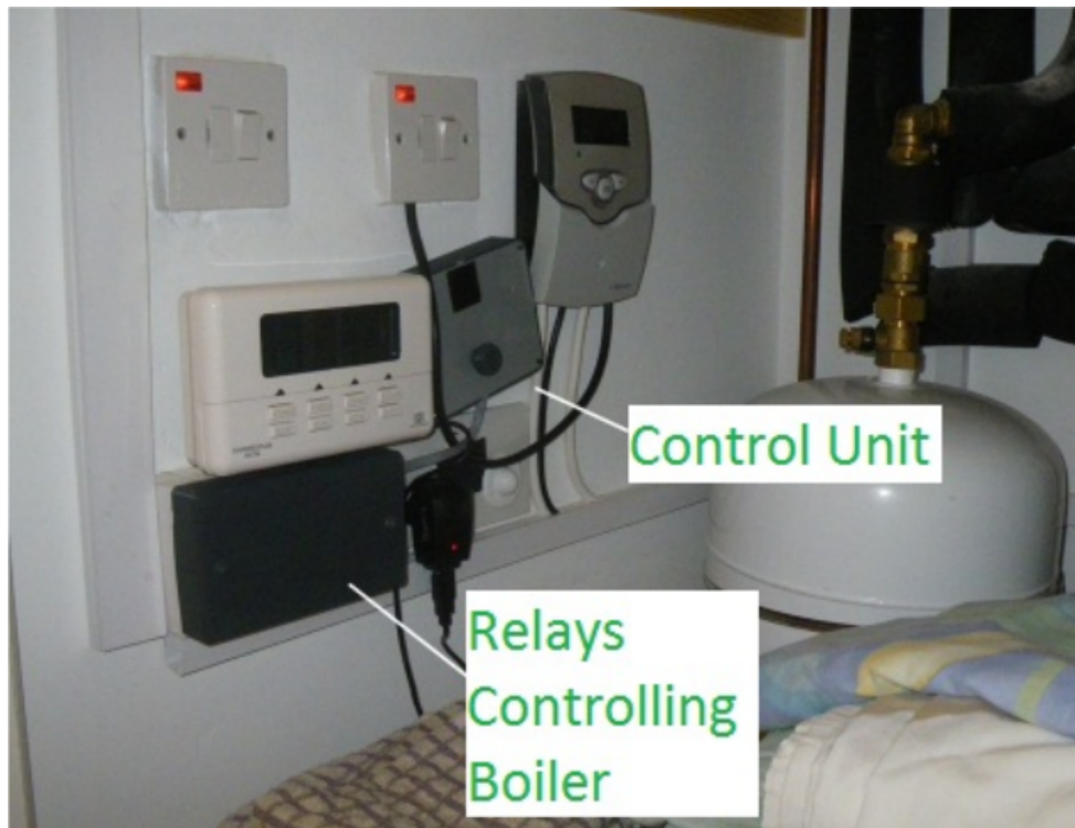
Figure 2.8: Control Unit from the U.K. wired into old boiler control circuitry [43].
