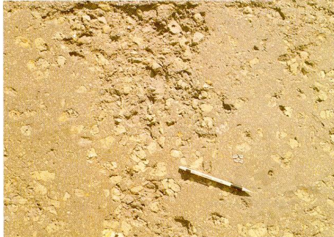
Figure 3-1 A typical example of raveling
