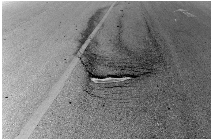
Figure 3-2 A typical example of other cracking
