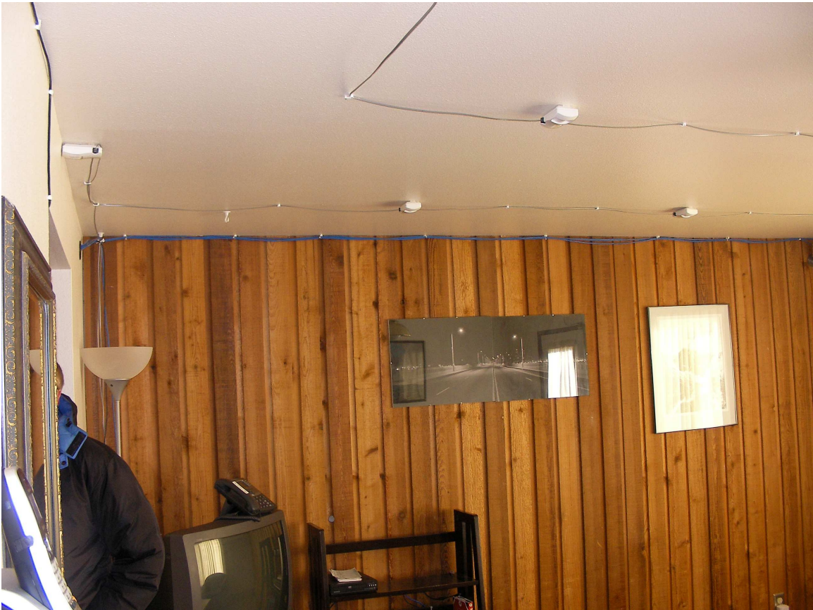
Figure 3.22: Sensors installed on the living room ceiling of the Kyoto testbed.
