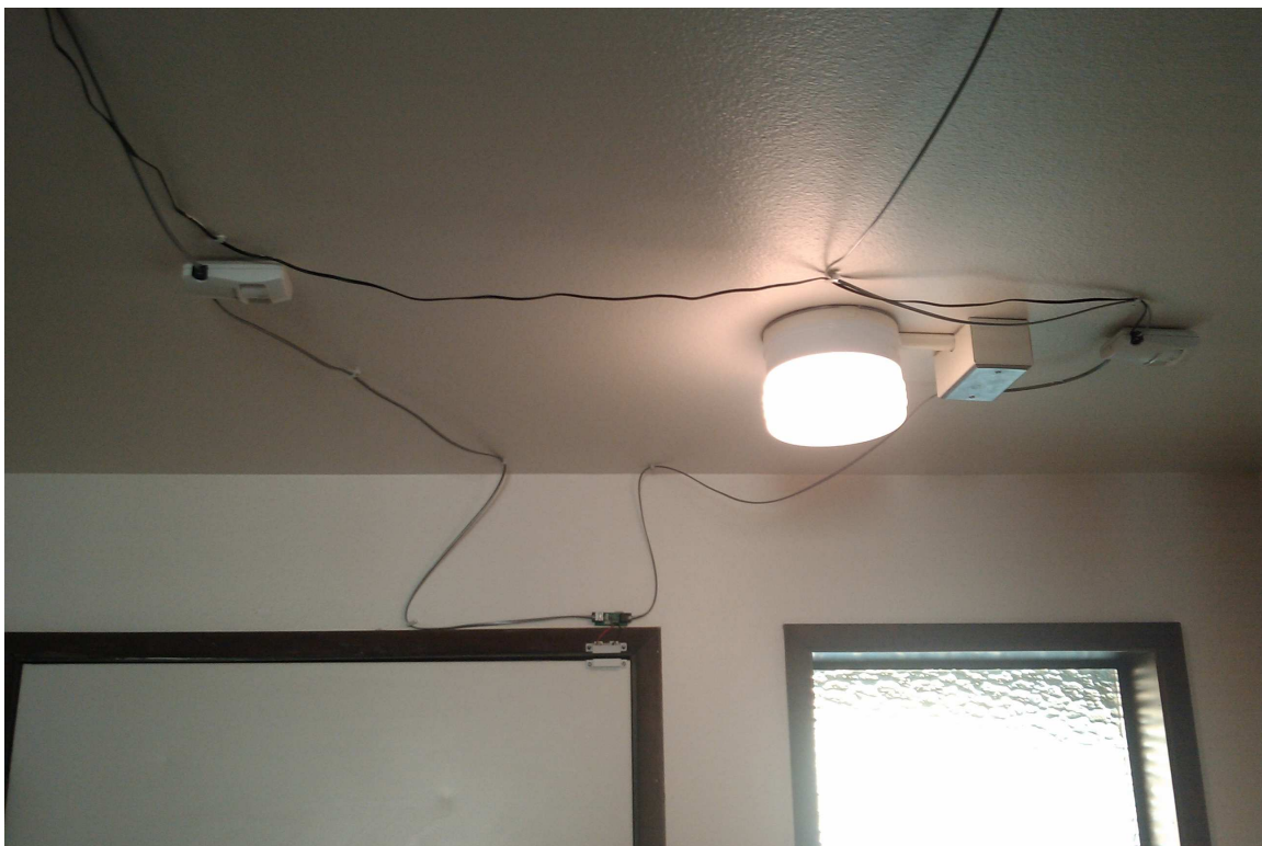
Figure 3.21: Sensors installed in the foyer of the Kyoto testbed.
