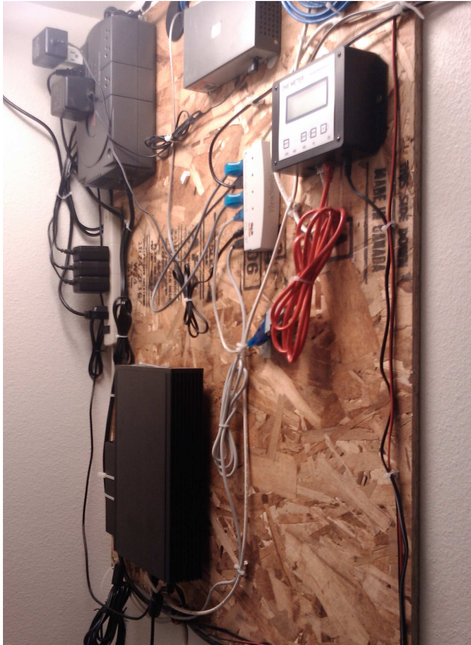
Figure 3.23: Central wiring board and server location for the Kyoto testbed.
