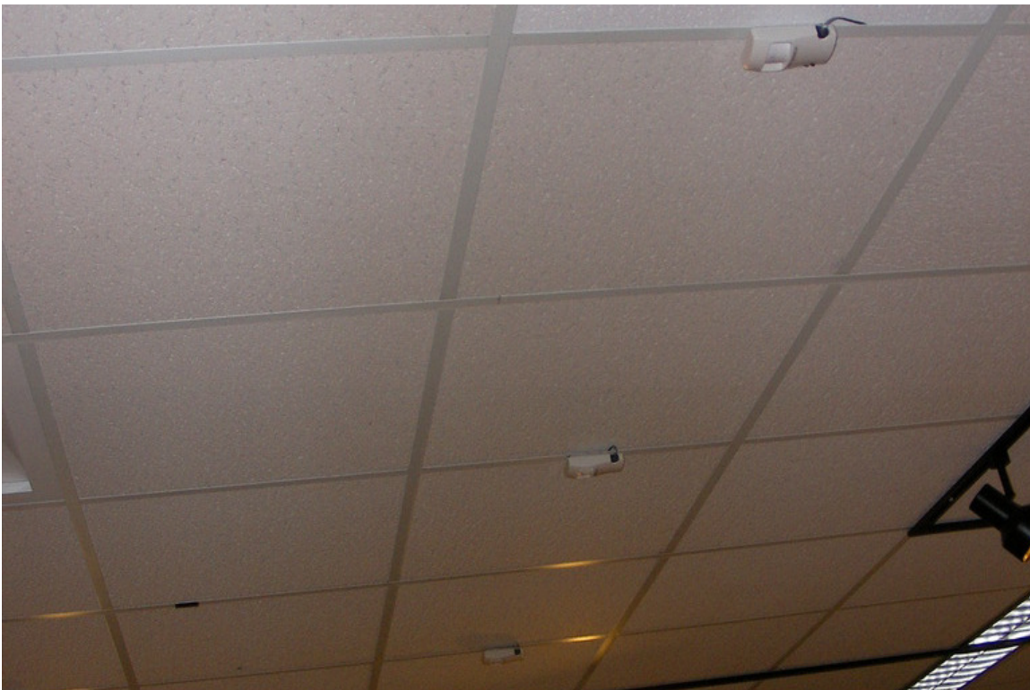
Figure 3.14: Example of the Tokyo testbed ceiling and sensor installation.
