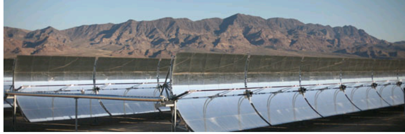
Figure 5: PTCs for Nevada Solar One [2]
