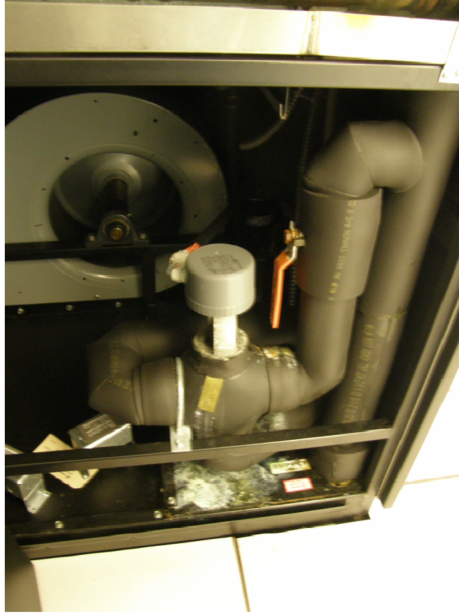
Figure A 28: Three-way valve within CRAC unit.
