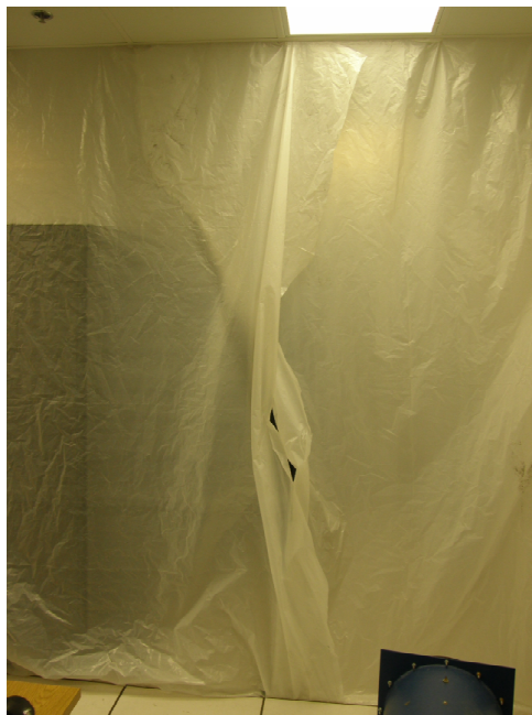
Figure A 30: Opening in polyethylene sheet to allow for passage of human operator.
