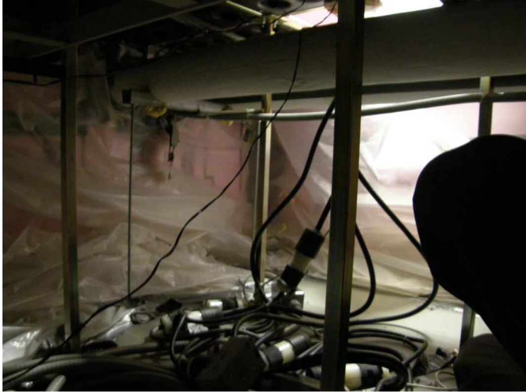
Figure A 39: Interior of control volume viewed from within raised floor plenum.
