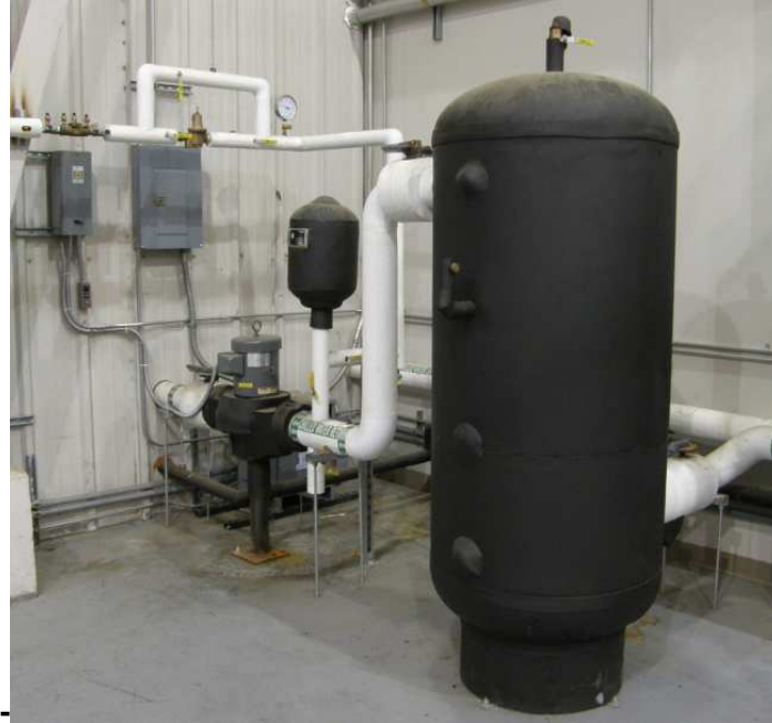
Figure A 2: Pump, tanks, makeup water, and associated piping in CEETHERM lab.
