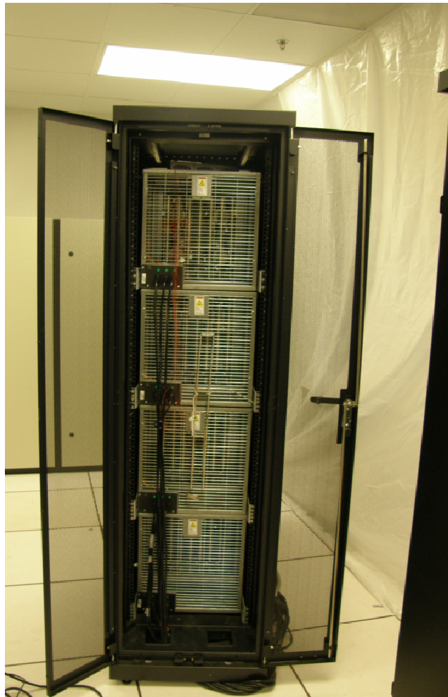
Figure A 8: Outlets of server simulator heater unit.
