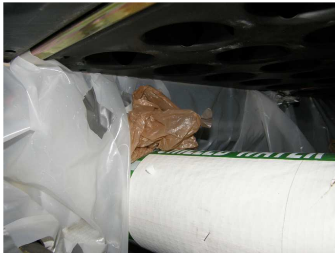
Figure A 32: Chilled water piping and cable trays were among the obstacles encountered while separating the hot and cold sides within the raised floor plenum.
