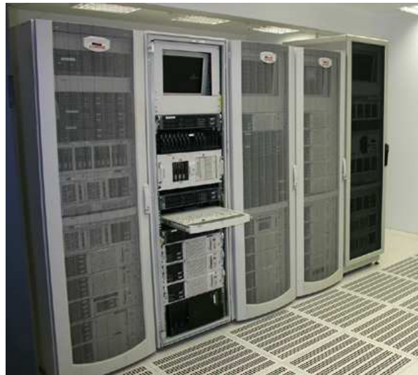
Figure 1.1-3: Server racks with clusters of rackable servers. [18]
