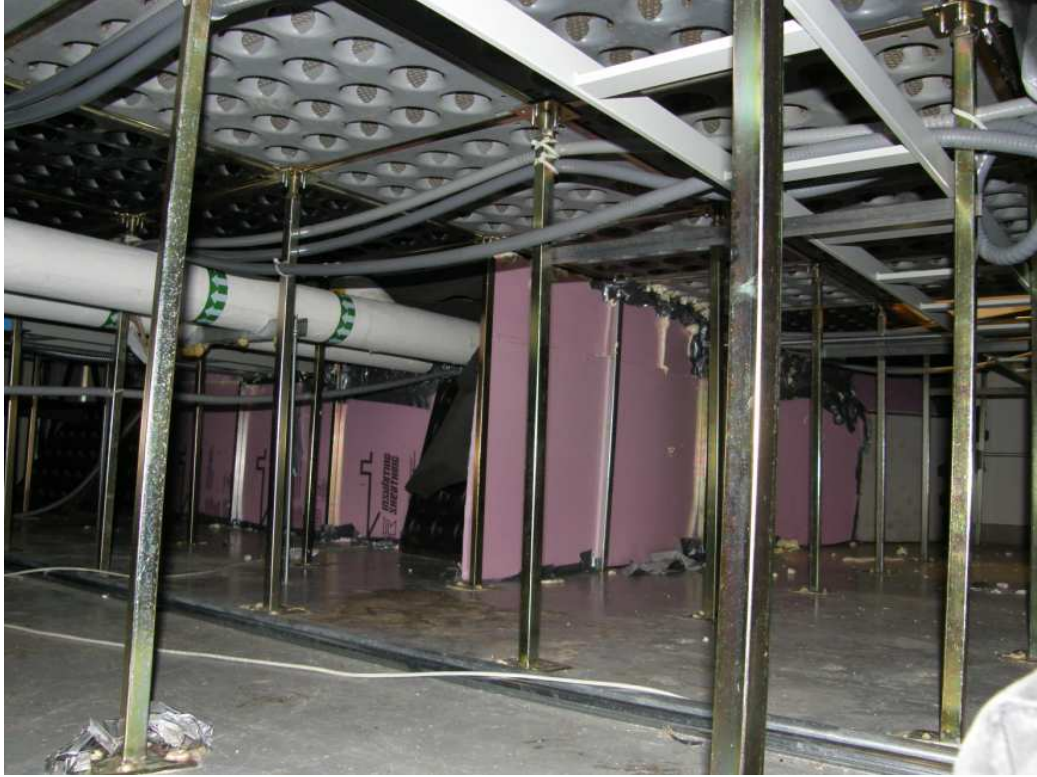
Figure A 38: Outside of control volume enclosure viewed from within raised floor plenum.
