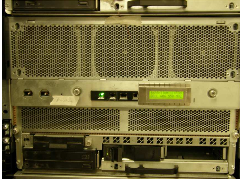
Figure A 10: Inlet to sample legacy server.
