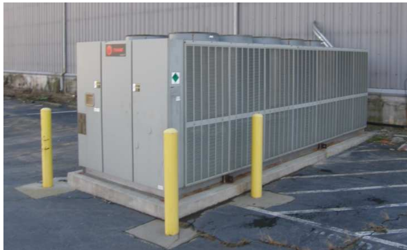
Figure A 1: RTAA-130 chiller at CEETHERM laboratory.
