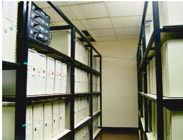
Figure 1.1-1: Perseus Beowulf compute cluster constructed from PCs and housed on Shelves. [15]
