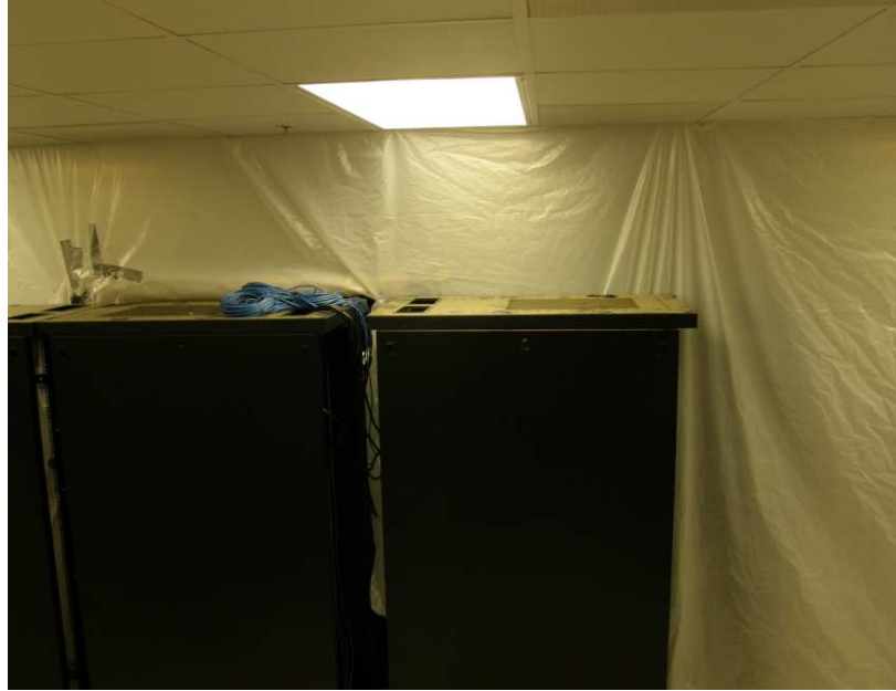
Figure A 31: Rack of servers adjacent to opening used to transfer said rack during transition between hot and cold sides.
