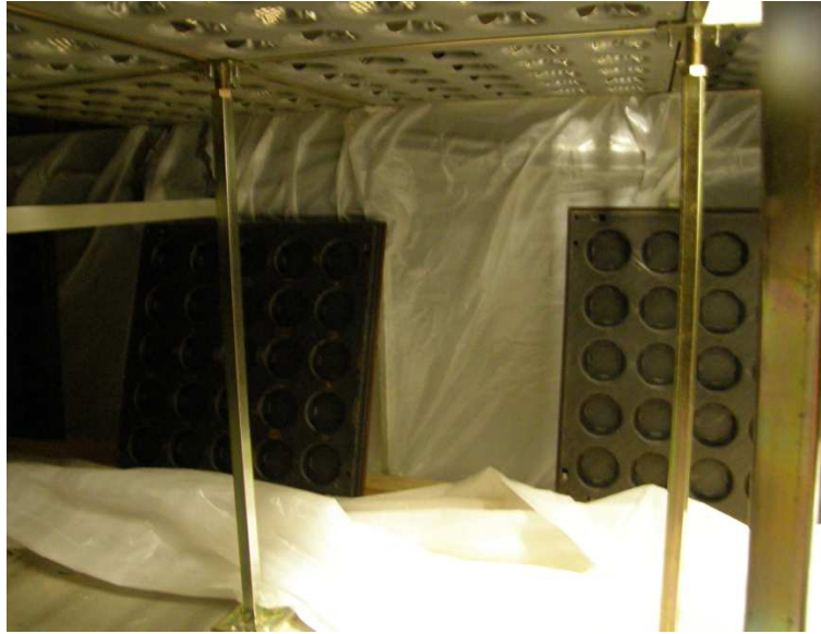
Figure A 29: Raised floor plenum divided by polyethylene sheeting to segregate air into hot and cold side.
