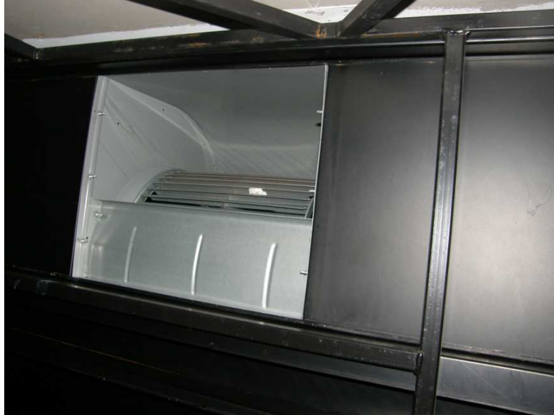
Figure A 24: Outlet of centrifugal fan beneath CRAC unit.
