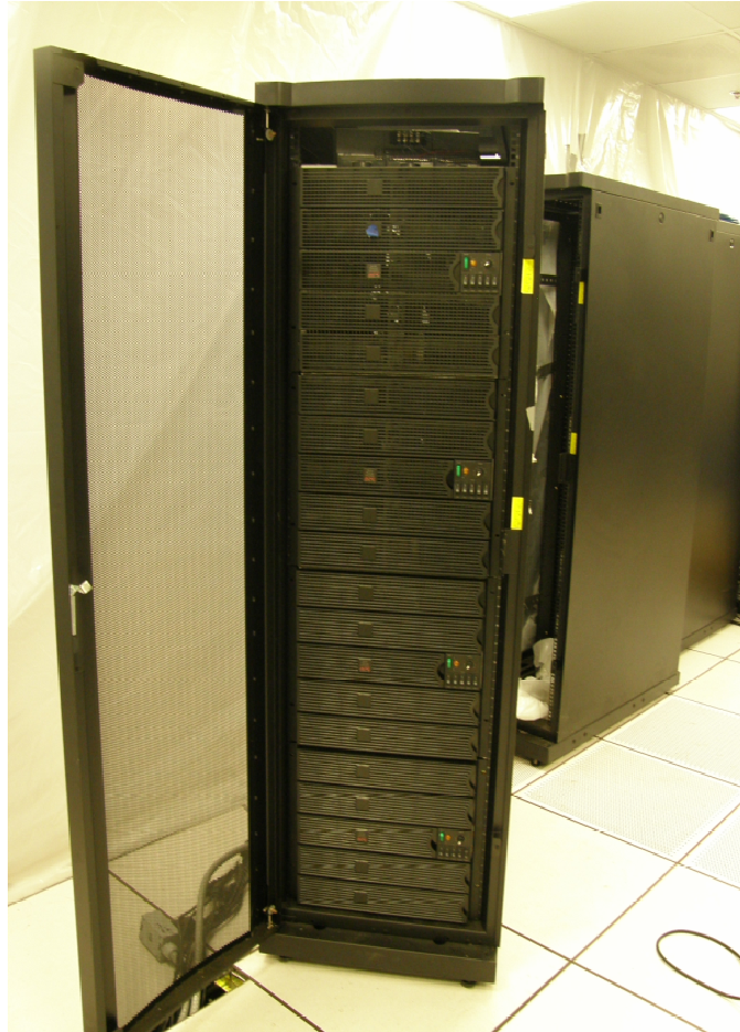
Figure A 7: Inlet to server simulator heater unit.
