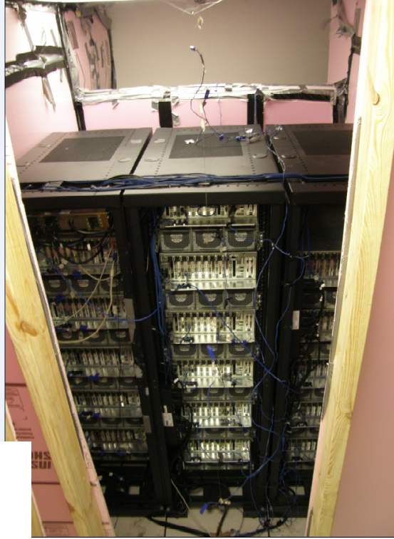
Figure A 36: Interior of control volume showing server outlets and return air path to air handler as viewed through opening in enclosure.
