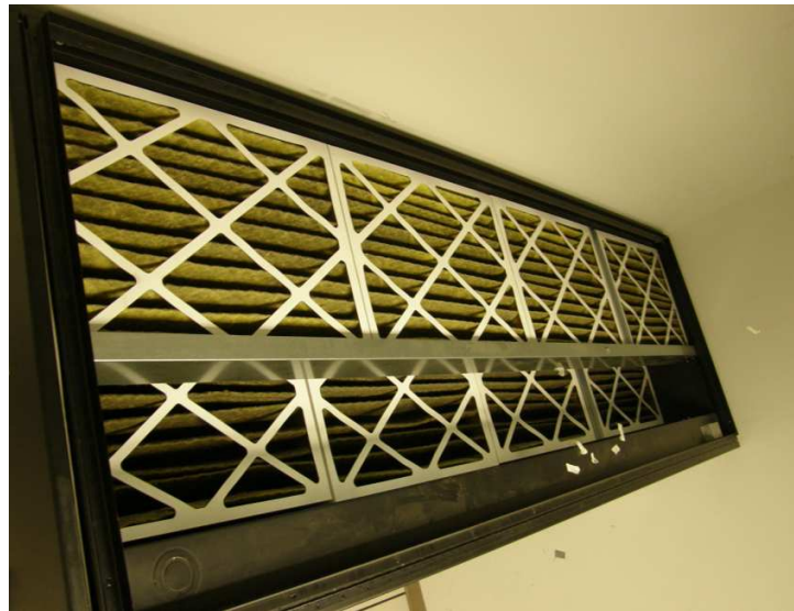
Figure A 22: Inlet of CRAC unit with filters.
