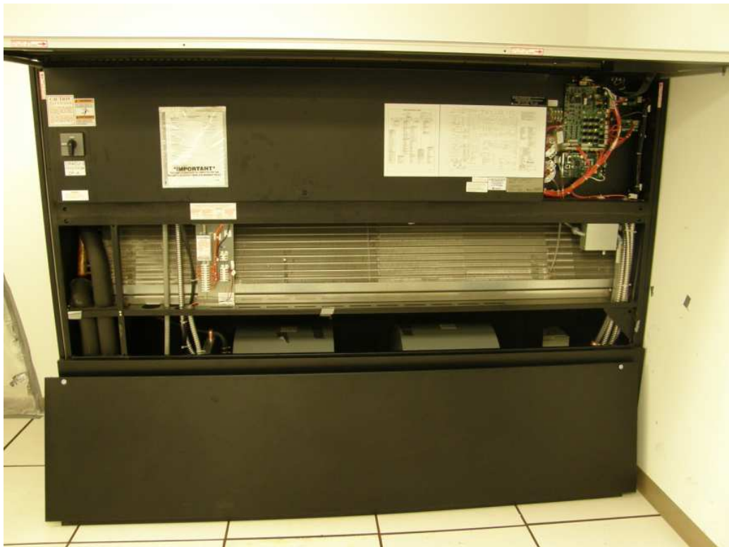
Figure A 25: CRAC with front panels removed to show heat exchanger.
