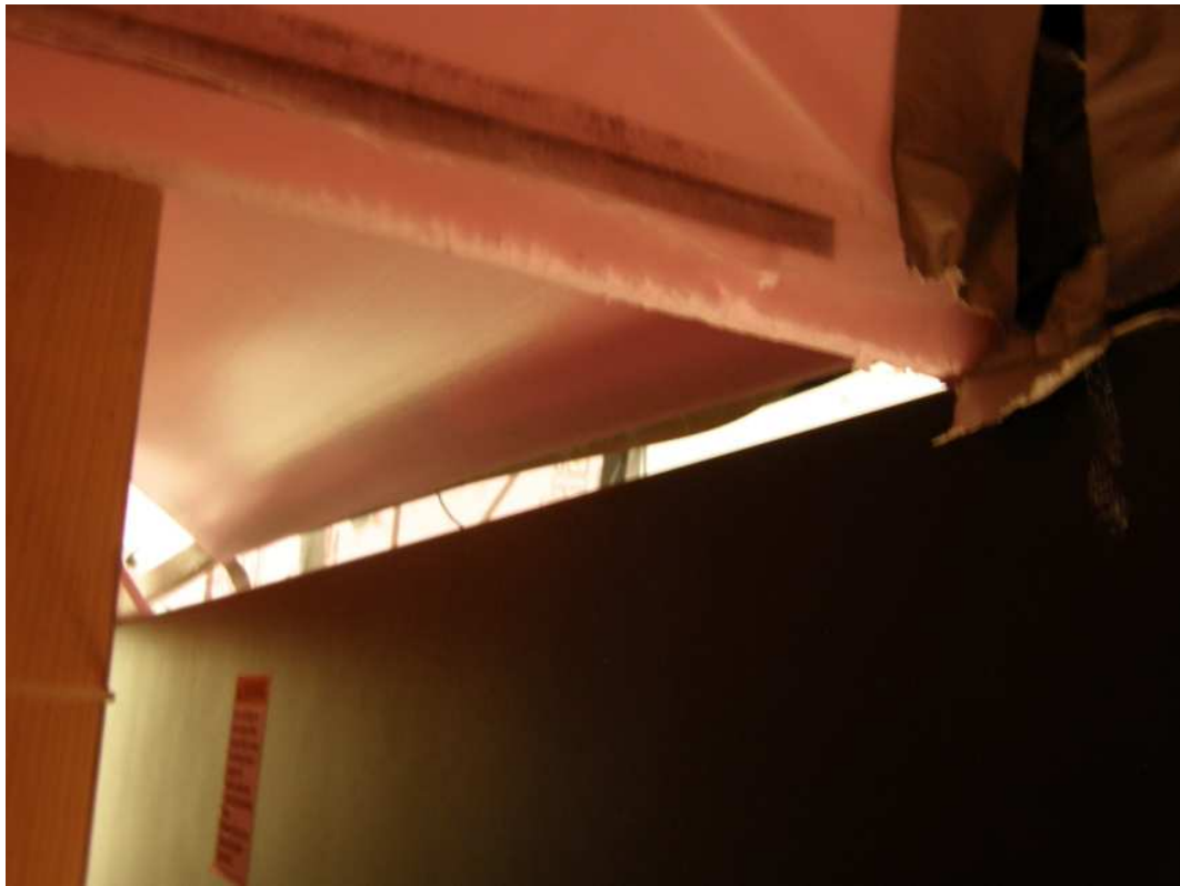
Figure 4.1-4: Gap in control volume enclosure caused by large negative pressure at air handler inlet requiring repair to obtain usable results.
