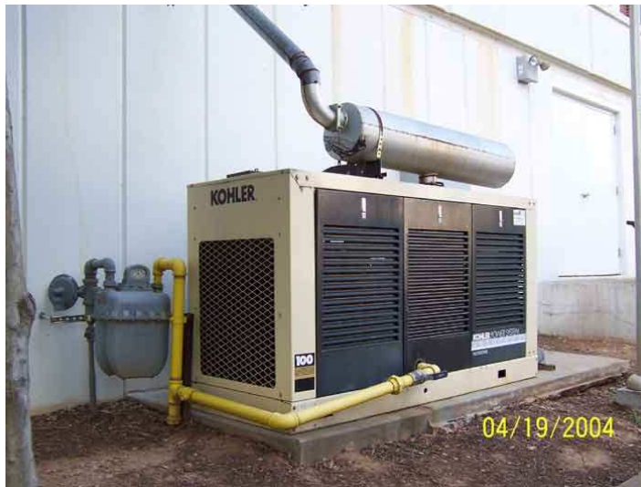
Figure 1.4-2: Emergency generator fueled by natural gas. [21]
