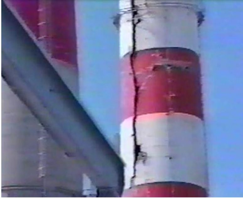
Figure 1-7: Structural damage to Turkey Point unit 1 exhaust stack [24].
