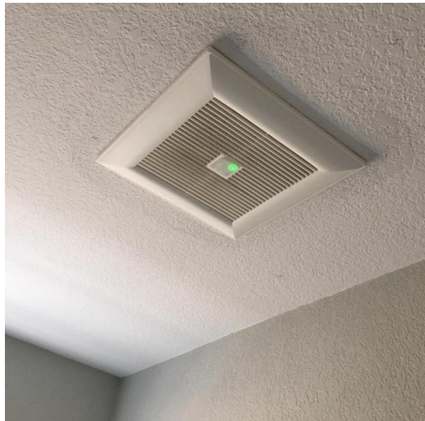
Figure 5. 2 An exhaust type mechanical ventilation system installed in a bathroom ceiling
