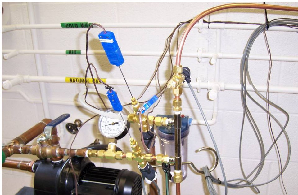
Figure 17: Snapshot of shell and tube heat exchanger with testing instrumentation
