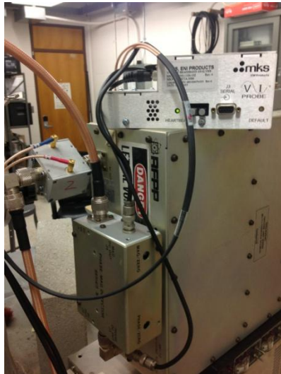
Figure 29: Alternate view of the Matching Network to show Bird Probe throughput and its connection to the analyzer.
