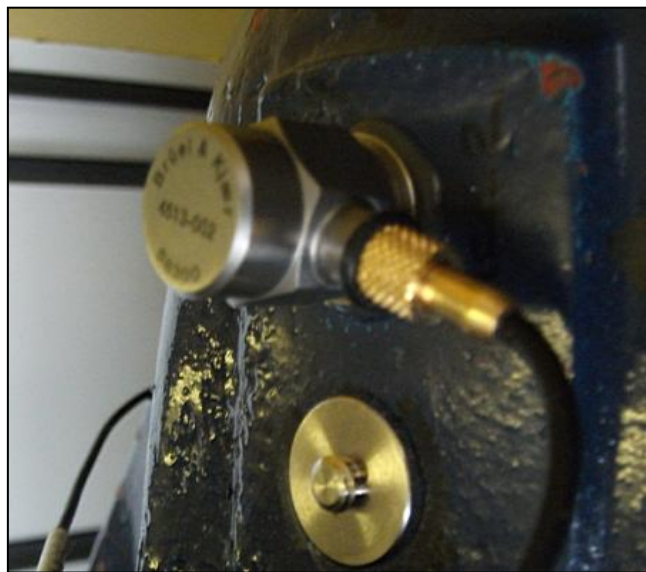
Figure 10: Photograph of an accelerometer on the gearbox high speed end
