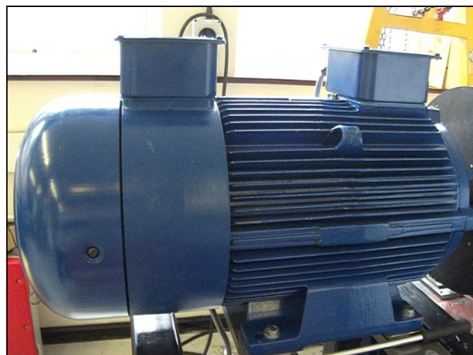
Figure 5: Photograph of the generator
