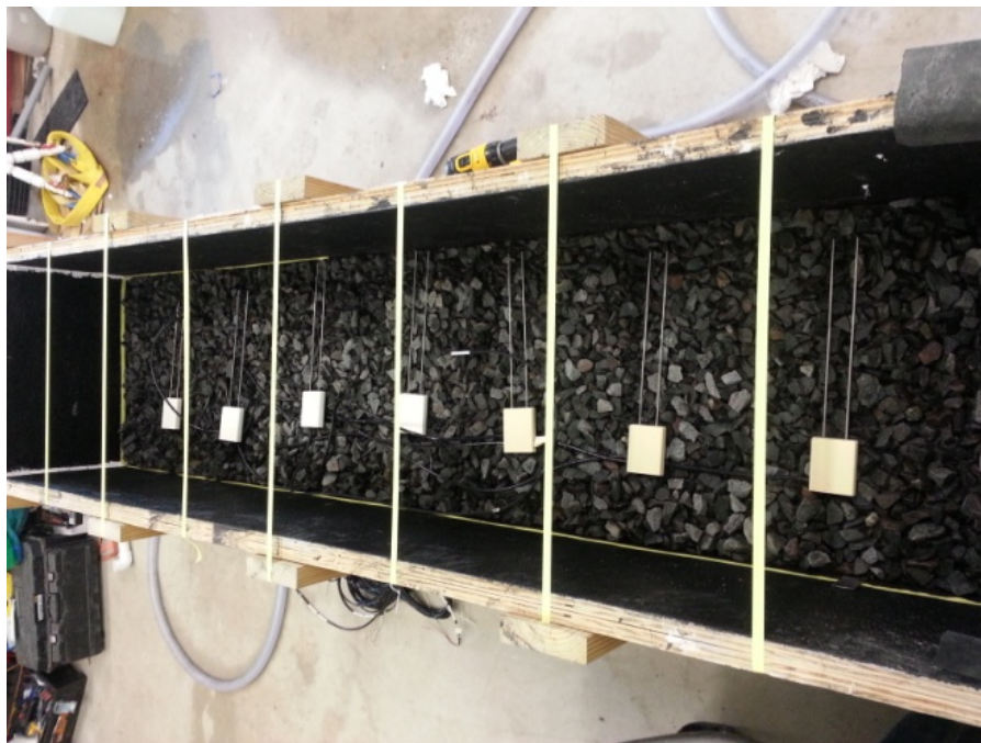
Figure 21: Arrangement of TDRs in the storage gallery
