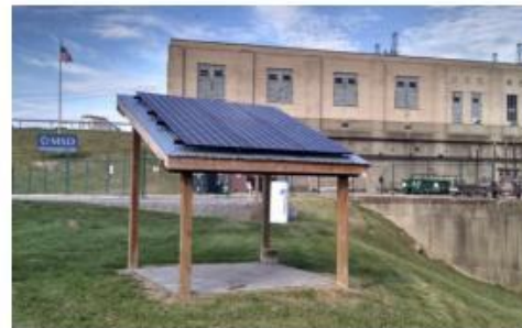
Figure 2. Solar panels for powering the water pump.
