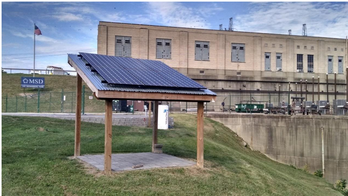
Figure 3.2 Panels for Powering Water Pump
